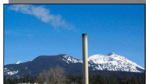
Stack from the Darby School Complex. A frigid day in February; all that can be seen is a small trail of steam.
